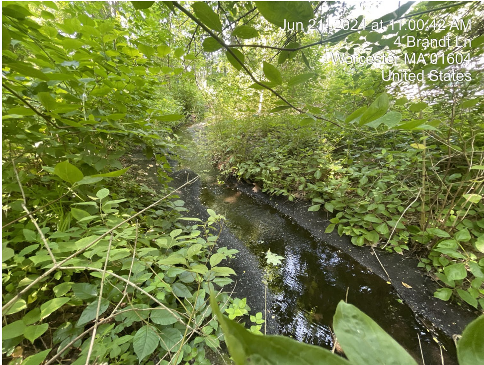
Paved swale for the intermittent stream (Impact Area 3)
